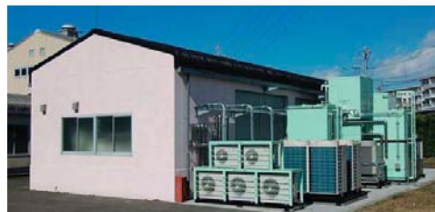
Environmental test facility for evaluation of hot water supplying heat pumps performance
