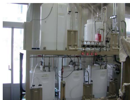
Chemical injection system
