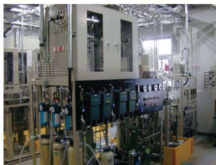
High temperature and high pressure loop system
