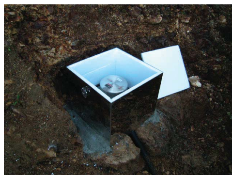
Strong-motion sensor installed on rock outcrop
