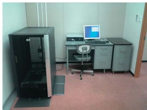
Backup server site at Akagi Testing Center
