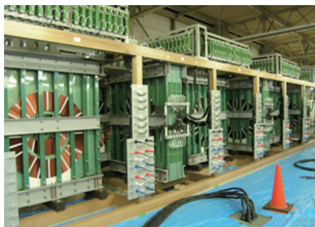
Photo 2 66kV transmission line emulator
