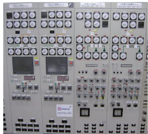
Generator operation panels
