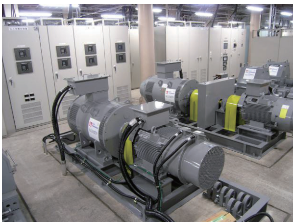
The full set of the thermal No.4 and 5 unit
