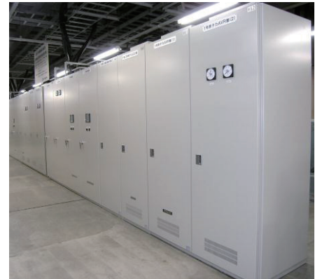
Nuclear unit control panel
