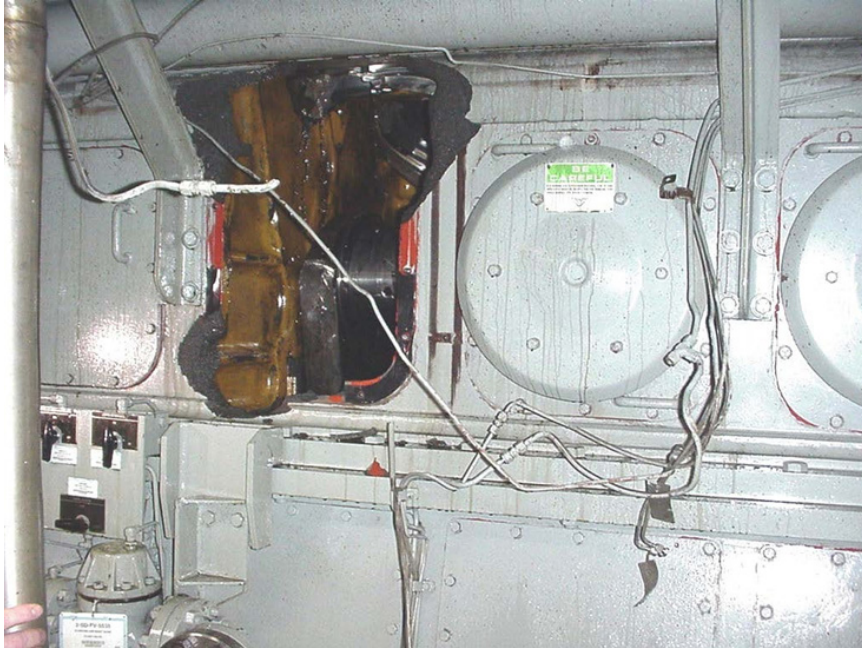
Figure 3.2-1: Image of the damaged Emergency Diesel Generator
